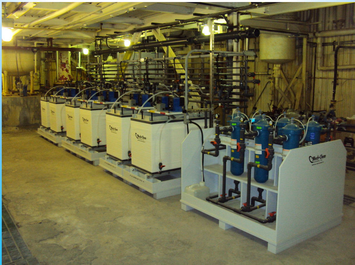
Picture of the filtration skid and six diffusion dialysis membrane modules. The system processes 1800 gallons per day of an acid leaching solution and recovers 90% of the hydrochloric acid for recycling to the ore leaching operation
