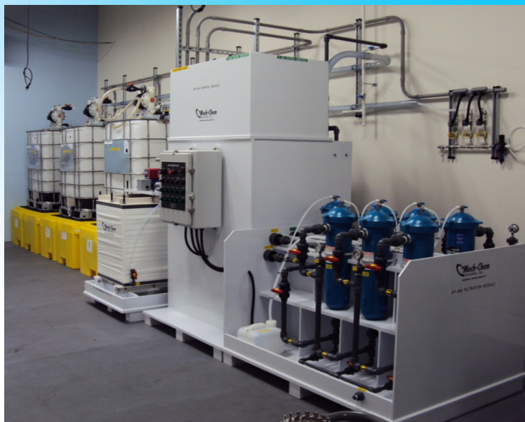
Picture shows a complete AP-300 system with filter skid and control module integrated with the clients feed acid and process tanks.
